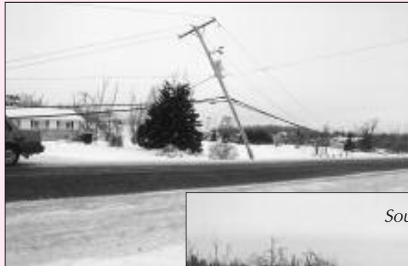
Steel towers in background are crumpled.
