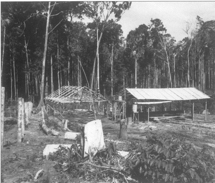
These structures will be used to dry cut lumber — essential buildings in this area of heavy rainfall
